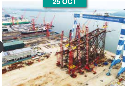
Successful Lifting of Kasawari Gas Development Project's Central Processing Platform (CPP) Jacket Top Panel Centre Box
